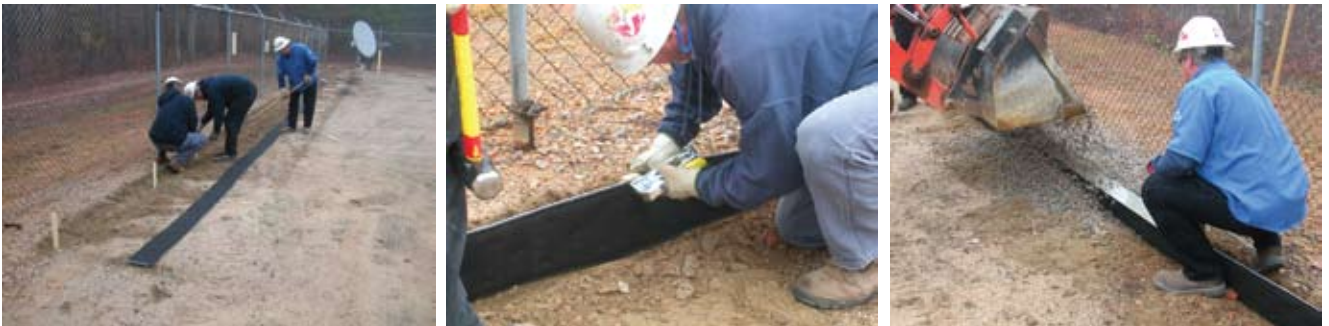
Substation install where subsurface is impervious
